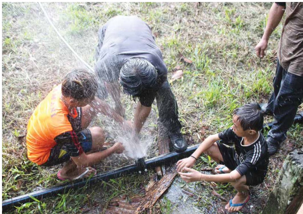
Kapt. Mohd Hafis and the team worked hard to ensure the water system was set up properly and well functions.
