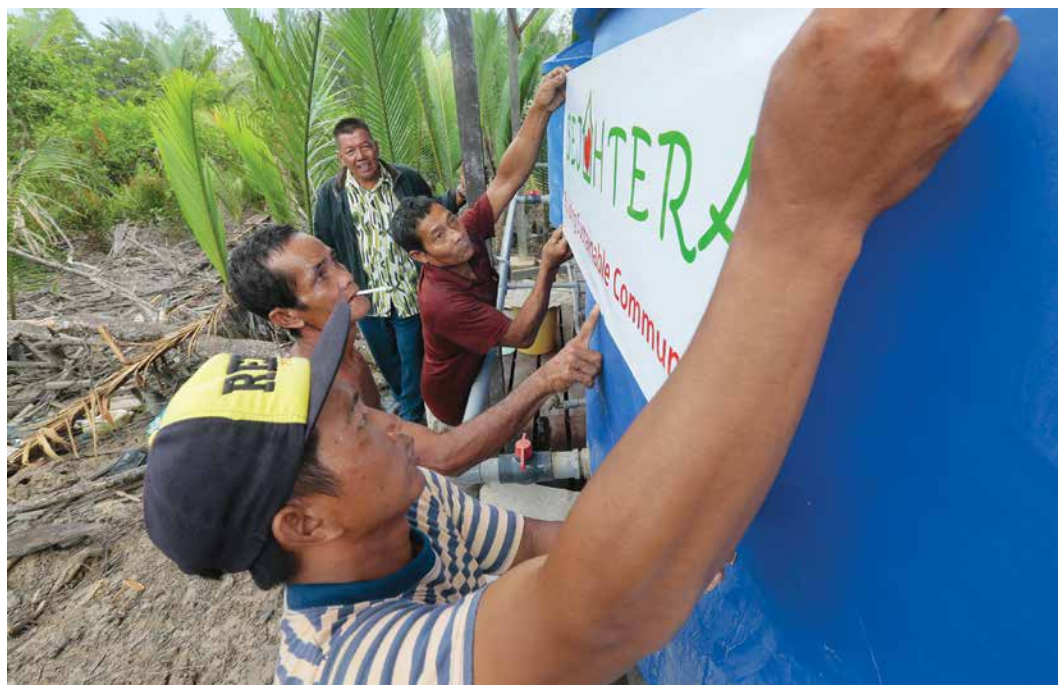
The villagers welcome the installation of the rain water-harvesting system in Kg Sebako.
