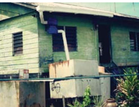
A house in Pulau Bruit fitted with a cyclone water filter system.
